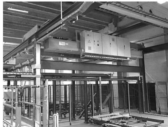
In the foreground: Transverse conveyor for anodised section being transferred from AMK3 to the store
