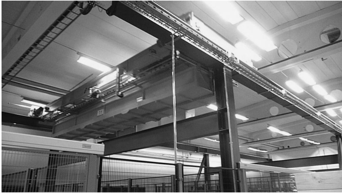
Automatic crane AMK3 in the anodising plant – the lowest of the crane transport levels
