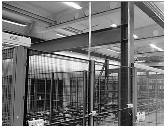
Under the crane track: Manual trolleys for moving racks to the jiggling areas in the anodising plant
