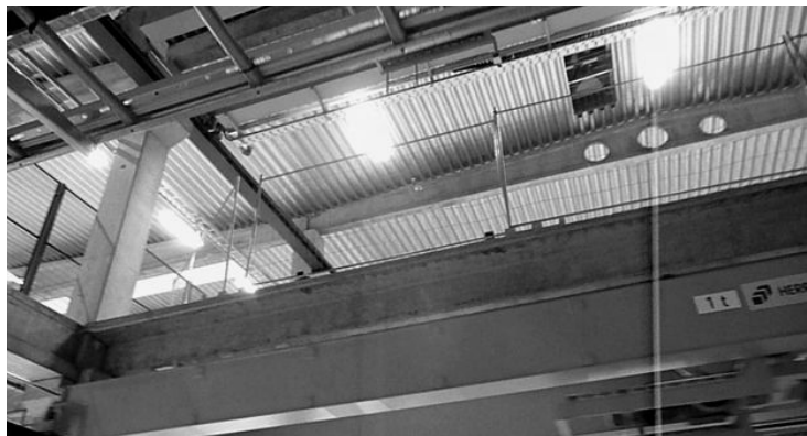
Cranes: AMK1 at ground level and AMK2 on the upper level of the store
