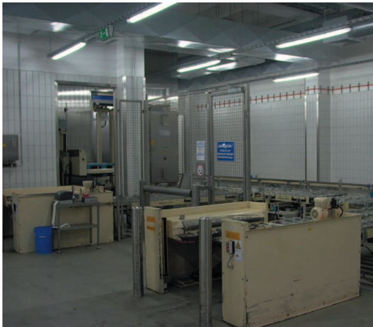
The goods, delivered by truck at ground level, are transfer by a lifting table into the transport system. Load supports not required are removed from the system directly next to the entry point.
