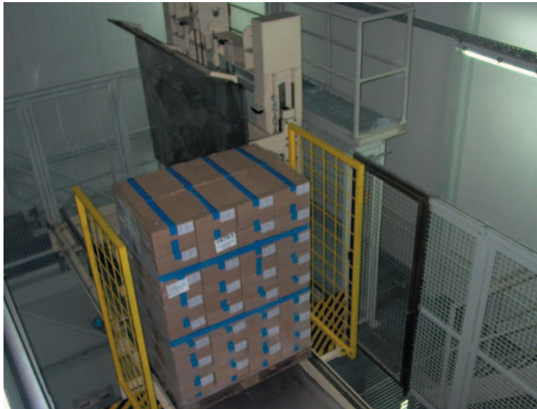
One of the two vertical conveyors takes the load unit to the vestibule of the store. Transfer from the vertical conveyor to the vestibule takes place at the upper level
