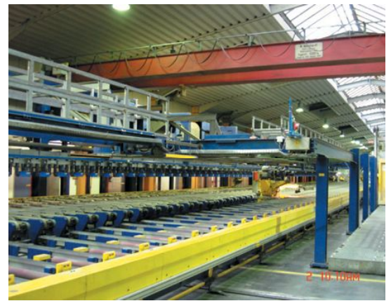
AMK 1 crane track above the cooling bed of press P1; on the right is the ageing furnace
